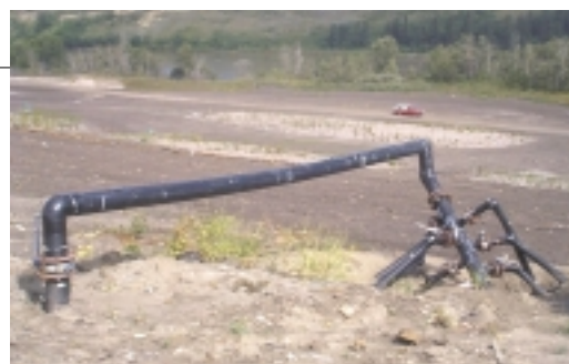
The City of Edmonton uses methane gas from its landfill to produce electricity for residential use.
